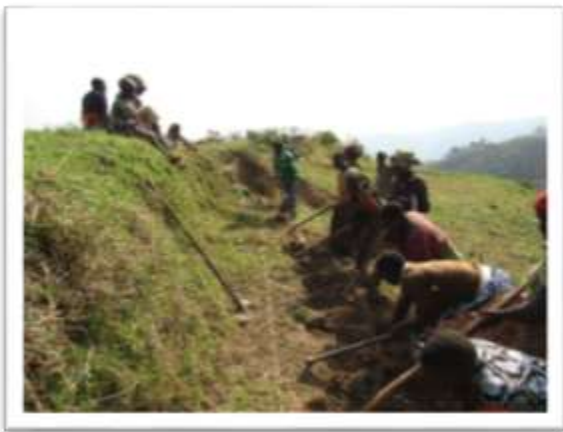
Farmers in Rwamahano construct a Fanya Chini terrace. With the heavy rains they're experiencing, farmers are witnessing the benefits firsthand.
